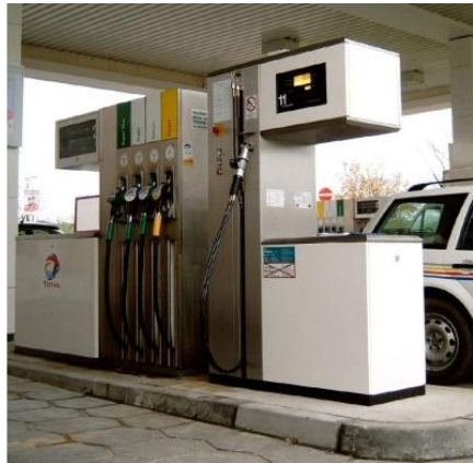
CNG filling stations
